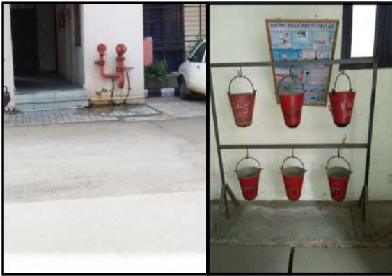
Fire Fighting Equipment
