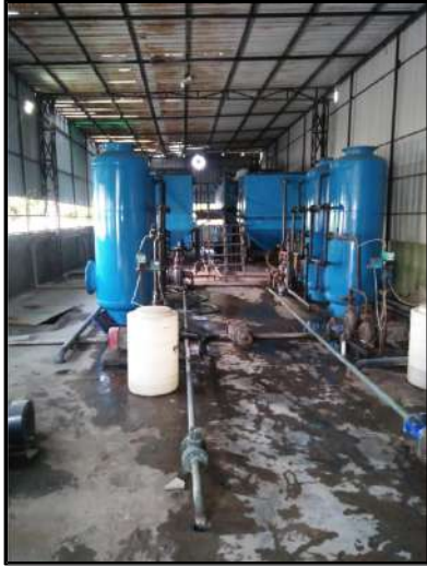
Sewage Treatment Plant
